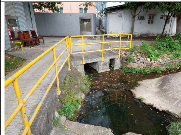
Plate 12 – Outfall of the existing 750mm U channel which receives discharges from the subject site at an existing watercourse
