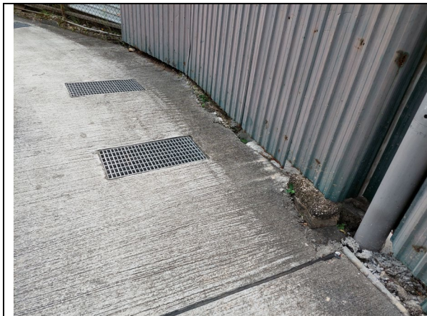
Plate 9 – Existing 750mm U channel receiving discharges from the subject site and running southwestward
