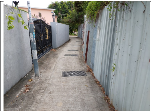
Plate 10 – Existing 750mm U channel receiving discharges from the subject site and running southwestward
