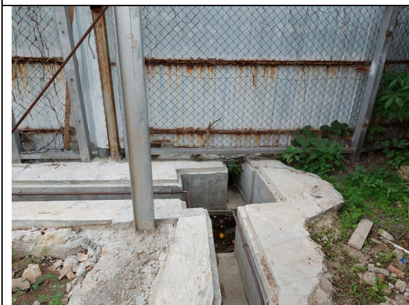
Plate 7 – Existing terminal catchpit with desilting facility at the southwest corner of the subject site
